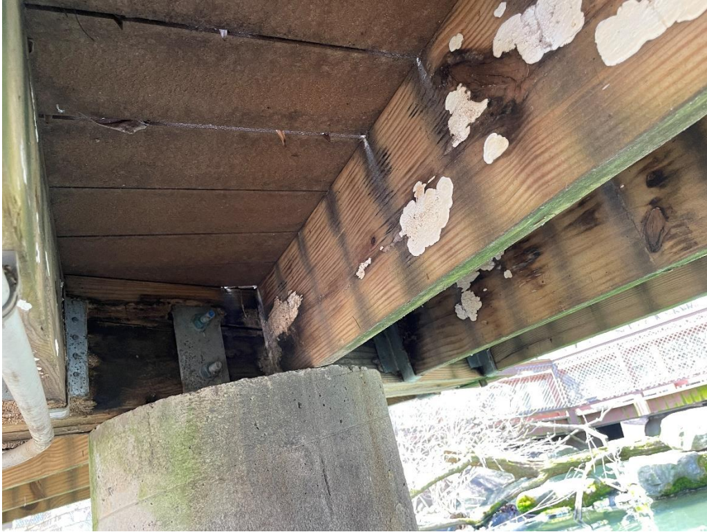
Photo 5 – Mold observed on the sides of rotted 2x10 joists
