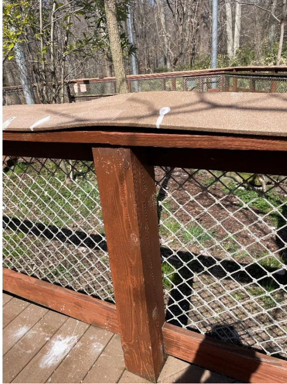
Photo 3 – Buckled composite railing topping material
