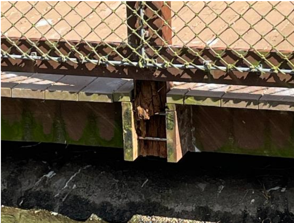
Photo 4 – Deterioration of 6x6 PT handrail post at base connection
