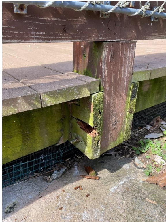
Photo 6 – Rotted 2x10 side members of built-up wood girder
